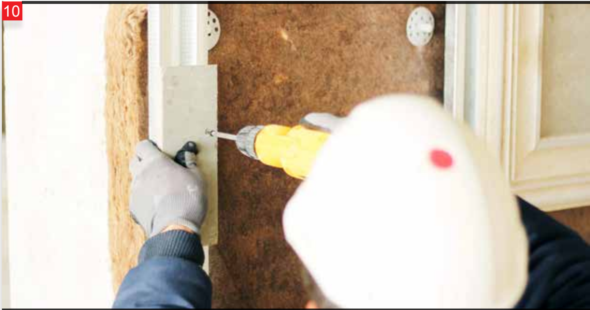
Balancing strips are placed on the middle sections of the area where the next panel will come.
