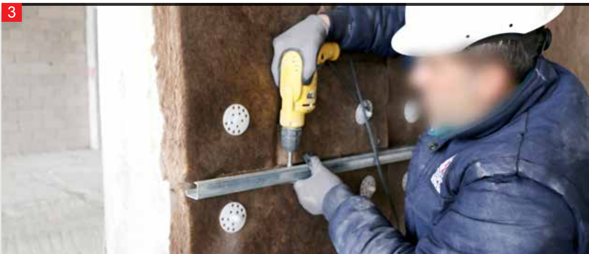
3 After fixing the stone wool on the wall surface the L profiles are attached to the L console with triphone bolts.
