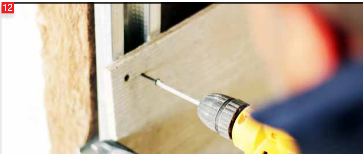
Screws are driven into the measured points as a guide to the overlapping panels.
