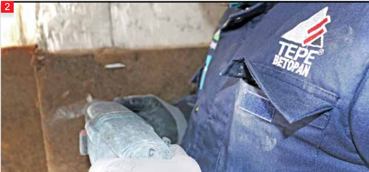
2 The necessary amount of stone wool is applied to the wall surface on the fixed L consoles.
