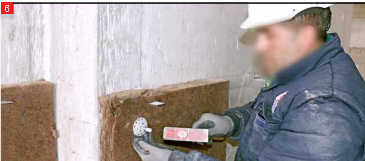
The applied insulation material is fixed to the application surface using parachute dowels.
